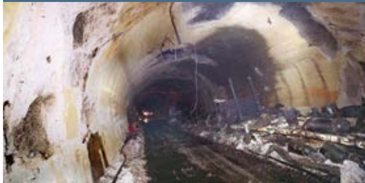
No fixed fire fighting system installed
